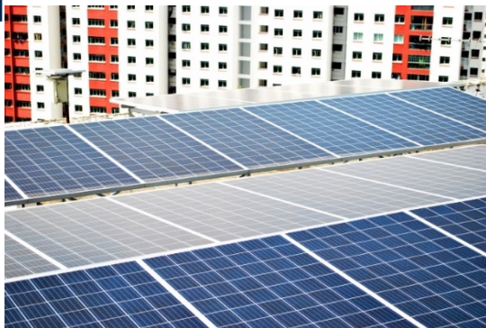
HDB rooftop PV
