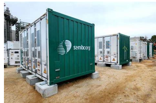
Energy storage project of Jurong Island
